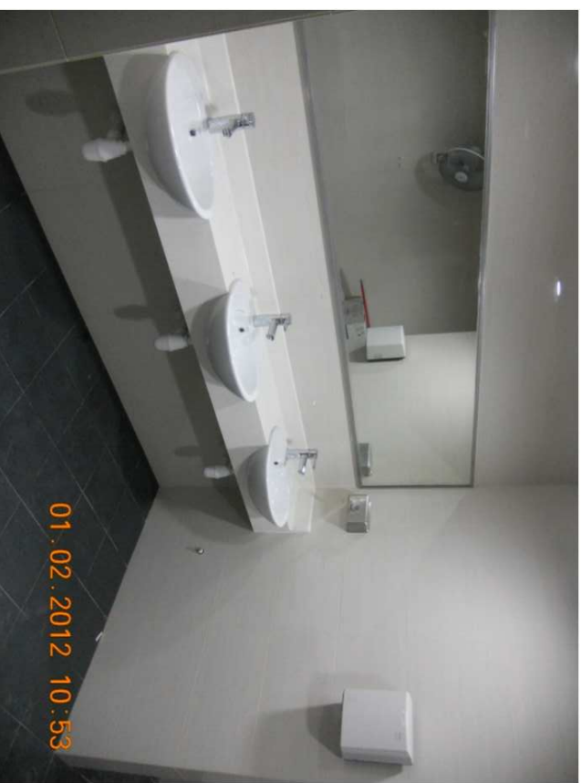
Toilets are completed with accessory
