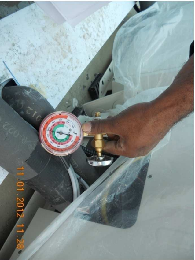
Pressure Test completed all condenser
