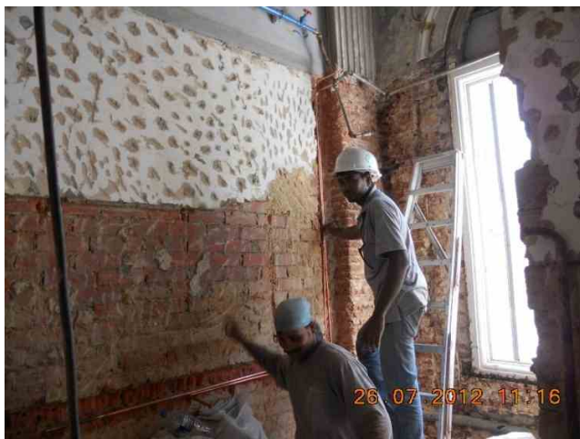
Removing of existing tiles and concealing of sanitary pipes are in progress at 2 nd STY toilet.
