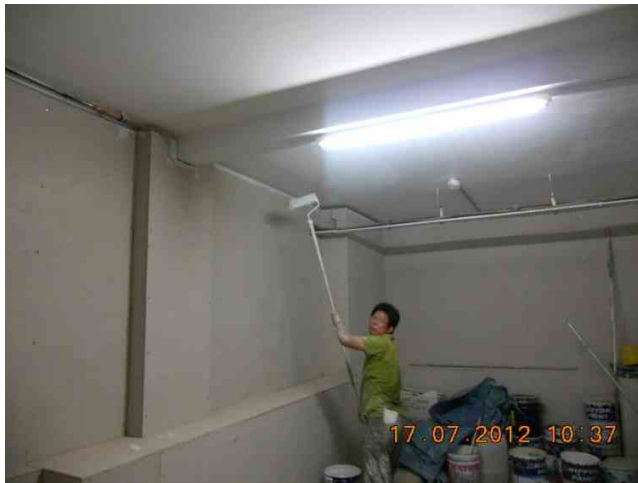
Ventilated wall completed except store room. Painting completed at the soffit of 1 st STY slab of basement.
