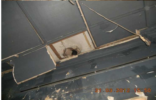
Asbestos ceiling expose after removing of 1 st layer ceiling
