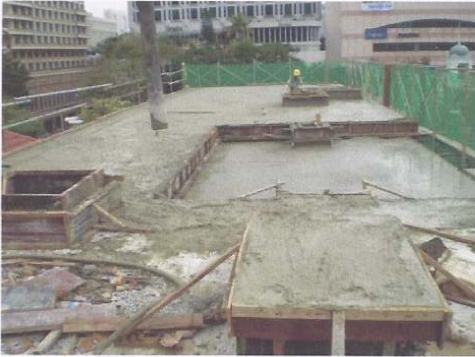
Casting of concrete to roof beams and slabs at gridline 2A-6A/A-B completed.
