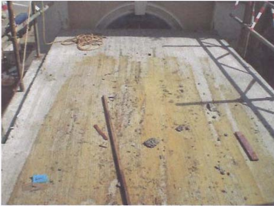
Formworks, rebar and casting of concrete to roof of link bridge completed.
