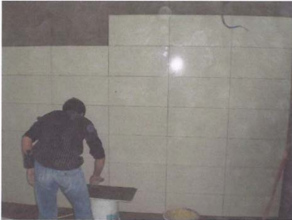
Laying of wall tiles to toilets / changing rooms at basement in progress.
