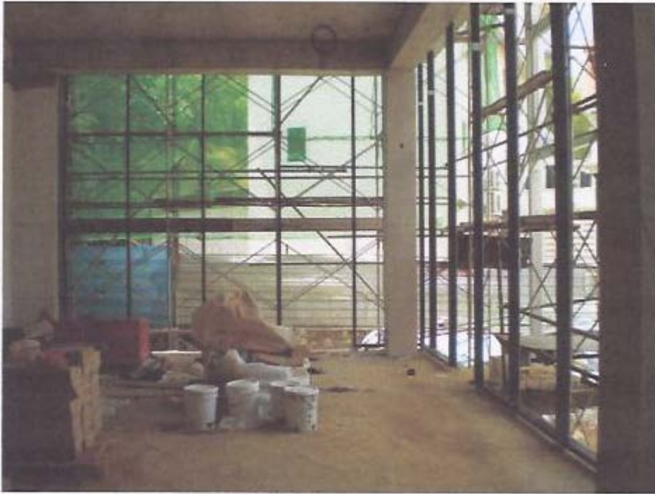
Installation of aluminum frames for curtain walls at 1 st storey in progress.
