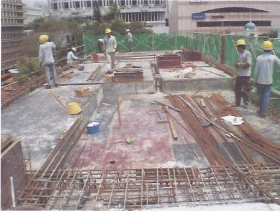
Formworks and rebars to roof beams and slabs at gridline 2A-6A/A-B in progress.
